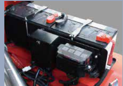
The integrated electrical box can be maintained easily
